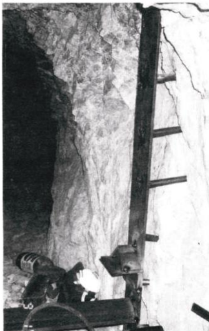
Marion Vittetoe anchors gates with heavy wall plates and large pins. These will be boxed in and concrete pouted into the frame for extra strength. Photo by Marion Vittetoe.
