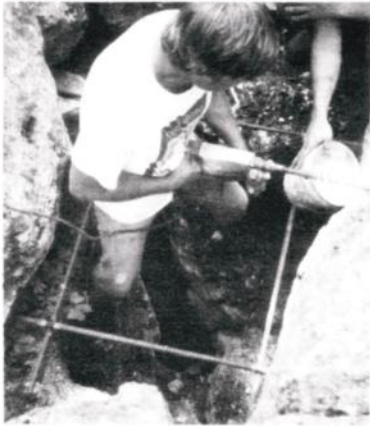
Mike Warton drills anchor holes with a hammer drill at Off Campus Cave, Texas.
